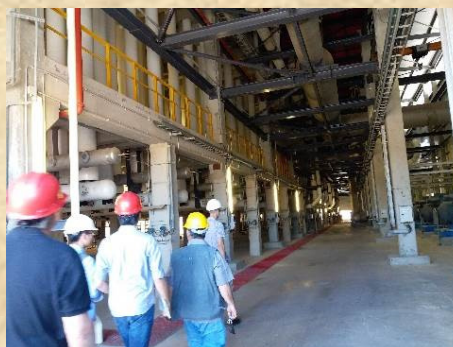
The multistage reverse osmosis desalination plant at Sorek
